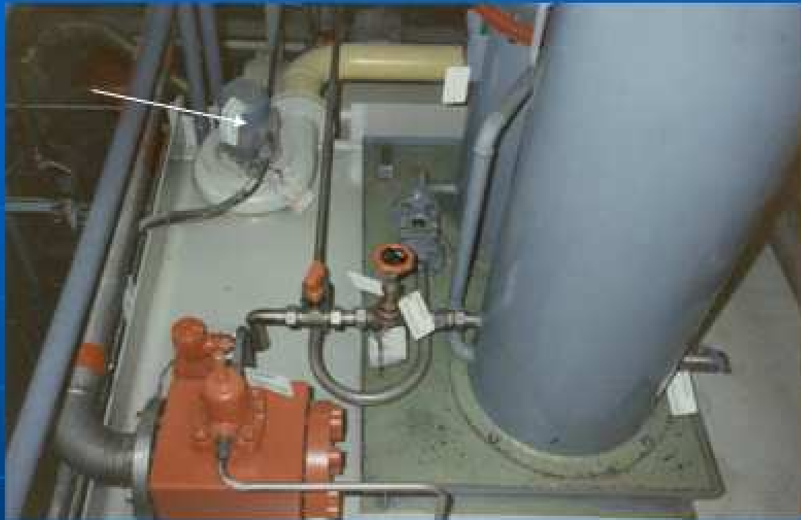
ABB Reservoir Top - Showing a PRV and the Vapor Extraction Fan
